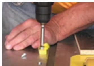
Use a Forstner bit to drill out the miter track to counter sink the bolt
